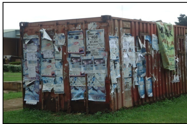
Plate 5. A defaced building and Container with bills. Source: Authors collection 2016.
