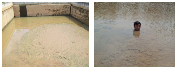
Figure 4. Sludge reservoir from water treatment plant of BOO Thu Duc water treatment plant and Tan Hiep water treatment plant.
