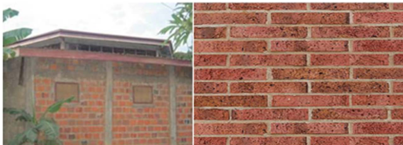
Figure 7. Examples of a poor and good workmanship. Source: Field study picture repository, 2016.
