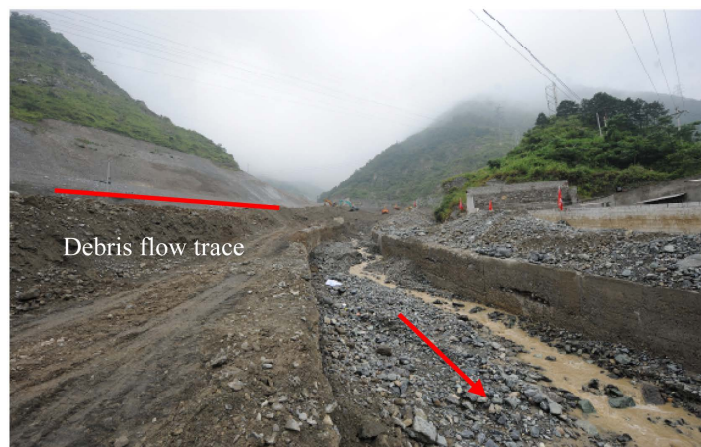
Figure 8. Debris flow buried drainage flume in the Hou Gully.
