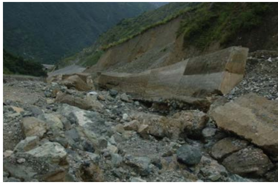
Figure 3. Destroyed prevention wall at the Hou Gully channel.
