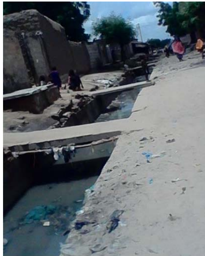
Picture 6. Open gutter and stagnating wastewater following the deposit of garbage (Bagalam district).
