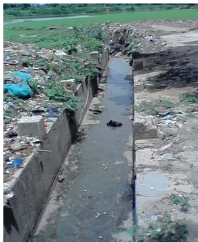
Picture 7. A drainage gutter wastewater jumping directly into Tabkin Dan Alatou (Assaou district).
