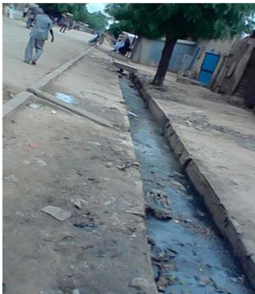
Picture 9. Poorly maintained gutter and filled with sand (saron gari district).
