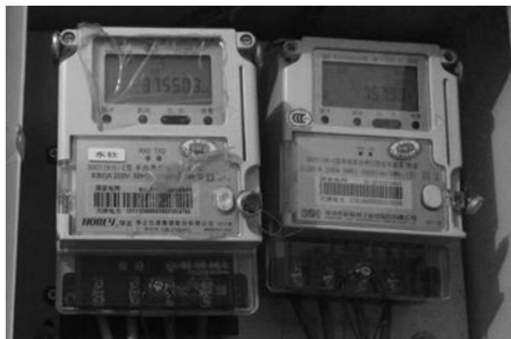
Figure 4. The two watt-hour meters installed in a household.
