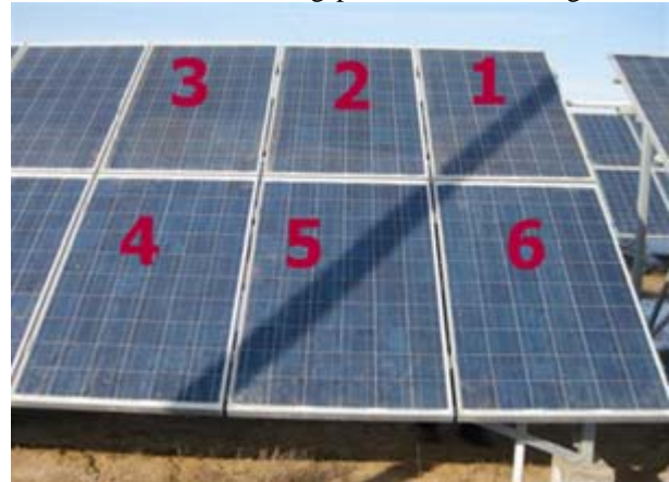
Figure 7. Wire pole shadows on the PV modules.
