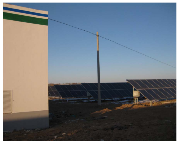
Figure 5. Power distribution room shadows on the PV module.
