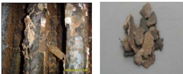
Figure 1. Corrosion schmutzband of the tube.
