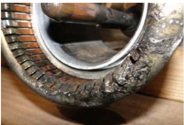
Figure 14. Circuit breaker contacts showing damage caused by electric arc.
