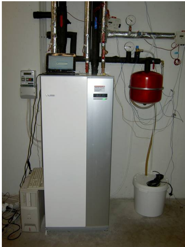
Figure 1. The heat pump in technical room of the building.
