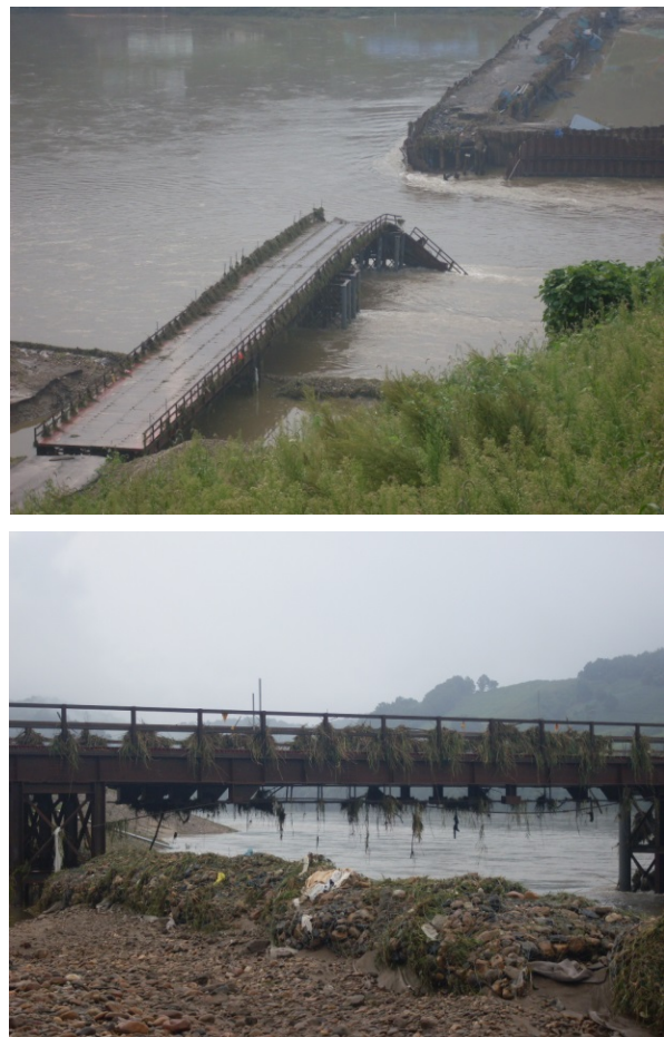
Figure 2. Temporary bridge for the construction of the flood control reservoir at the study area.
