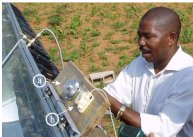
Figure 2. Two of the installed pyranometers: a) CMP11 LU and b) new SRS1000
