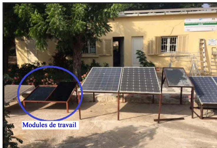
Figure 1. Photovoltaic field at CERER.
