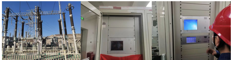
Figure 5. Substation data collection site.
