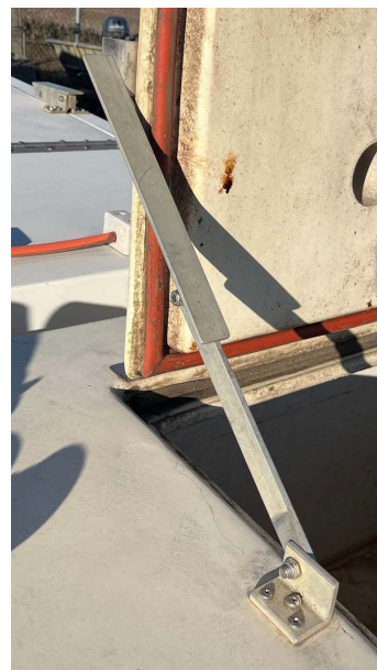
Figure 2. Photograph of folding lid stay hinge locked in an open position.
