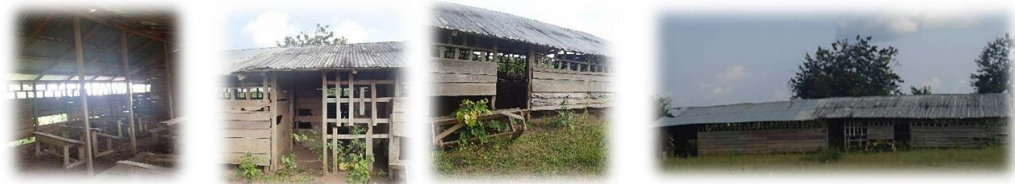
View of the condition of the Belamboké school in 2018 at the time of the study.
