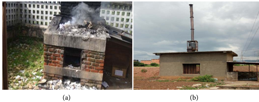
Figure 4. Incinerators used to treat solid medical wastes in 12 HCFs in Bujumbura, Burundi. (a) Low temperature incinerator (<math><300^{\circ}\text{C}</math> - <math>400^{\circ}\text{C}</math>) used by 11HCFs and (b) Medium temperature incinerator (<math>700^{\circ}\text{C}</math>) used by 1 HCF.
