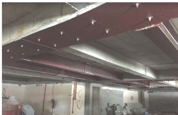
Figure 10. Actual photo Reinforcement of reinforced concrete beam bending resistance by gluing steel plate.
