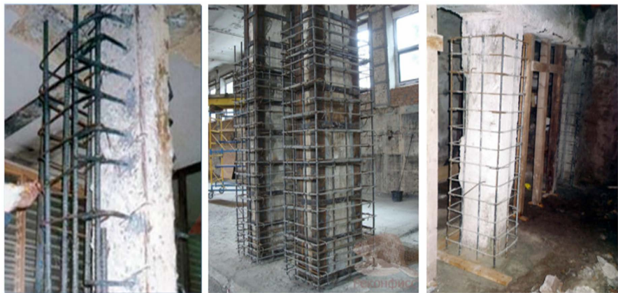
Figure 8. Actual photo reinforcement by increasing column cross section size in project, Hanoi, Vietnam.
