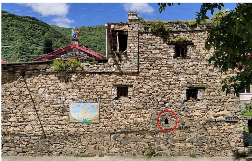
Figure 3. The ventilation hole in the ground floor (source of the picture: the author shot).
