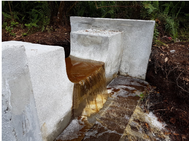
Figure 9. The design of check dam established at Parit Pulau and Parit Gantung.
