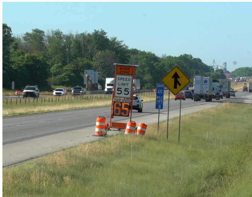
Figure 1. Radar-based speed limit sign with motorist speed feedback.
