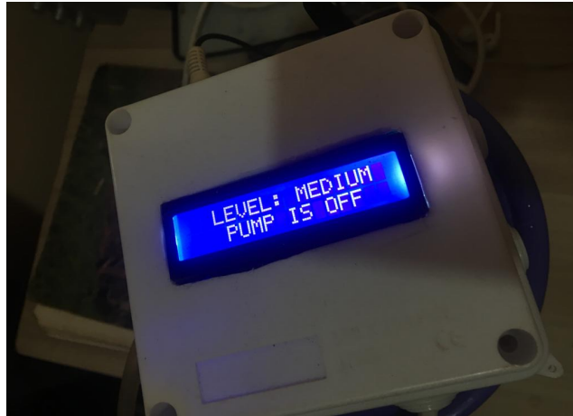
Figure 5. Indication of the submersible pump being OFF.
