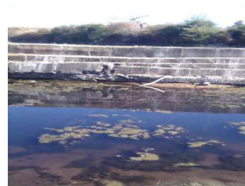
Locally known as ka weir kanini or ka dambwa -made of sand bags or concrete to create an embankment and conserve or harvest rainwater.
