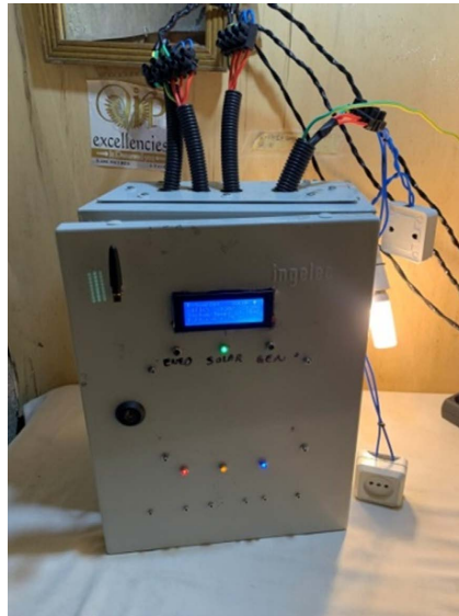
Figure 17. Exterior view of complete ATS system.
