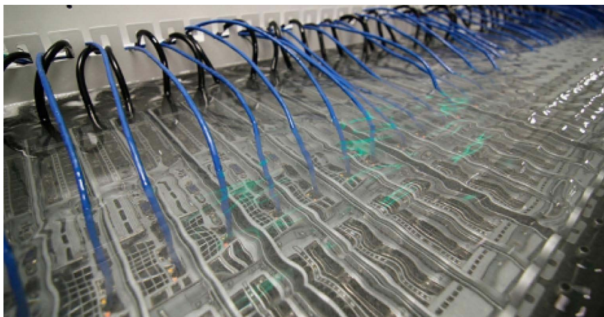
Figure 2. Bath immersion cooling for blade servers [16].
