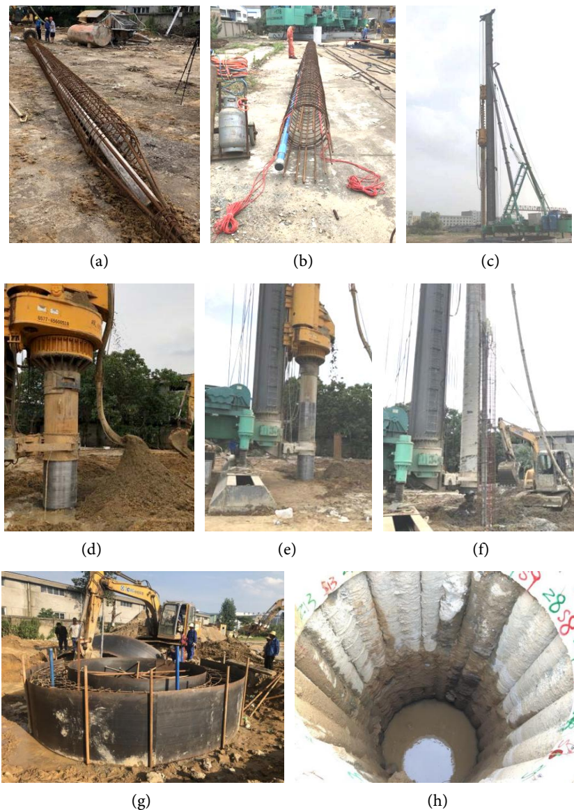
Figure 2. Construction site of bite pile. (a) Pile bottom—cone, (b) pile top—Circular, (c) drilling rig—48 m high, (d) Earth squeezing, (e) pressure pouring concrete, (f) inserting reinforcement cage, (g) Pouring crown beam, (h) pile group.
