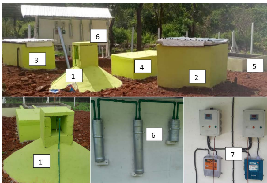
Figure 1. Overview of the 2nd Methanizer of the BRIN FOUNDATION. 1: Methanizer; 2: Manual feeding tank; 3: Automatic feeding tank; 4: Expansion tank; 5: Retention tank for digestate (compost room); 6: Biogas filtration and purification system; 7: Temperature sensors (digester and digestate).
