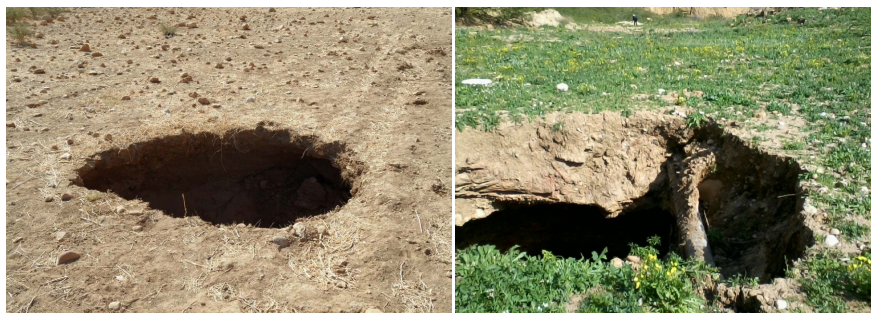
Figure 7. Collapses of ceilings of cavities which were created by pumping of Triassic and Jurassic salty water ( \sim 15,000 \mu\text{S}/\text{cm} ) and replacement by fresh water ( \sim 1,000 \mu\text{S}/\text{cm} ) resulting in additional dissolution of evaporates and formation of underground cavities.
