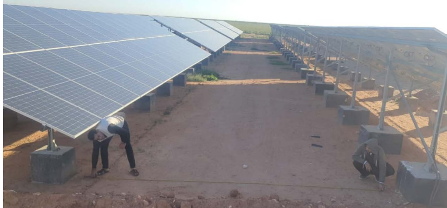
Figure 4. Each array contains two strings and panels.
