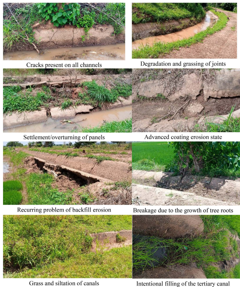
Figure 5. Some of the most recurring degradations on the irrigation network of the perimeter.
