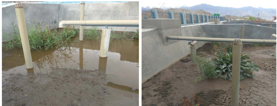
Figure 6. Faecal Sludge Treatment Plant in Leh using Phragmites .
