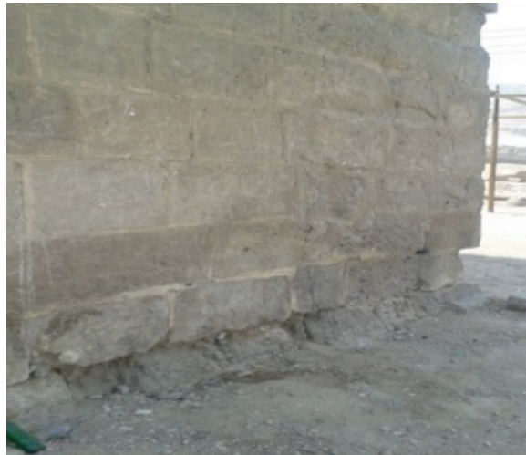
Figure 4. Continuous deterioration action resulted from efflorescence and salt crystallization.
