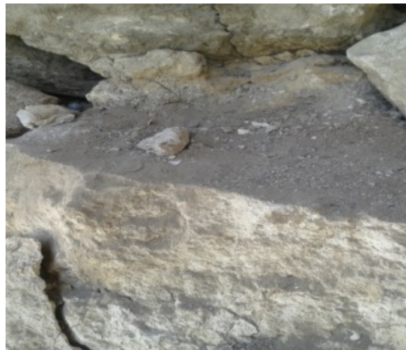
Figure 5. Foundations affected by ground water.
