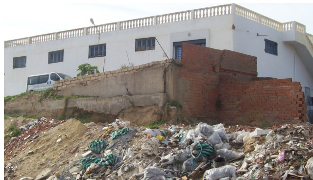
Photo 1. Fracturing and detachment of the wall located on the edge El Wadi Ain.
