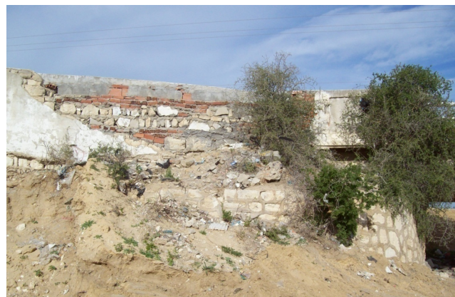
Photo 2. Fall of a portion of the wall at the bridge El Kebir wadi.
