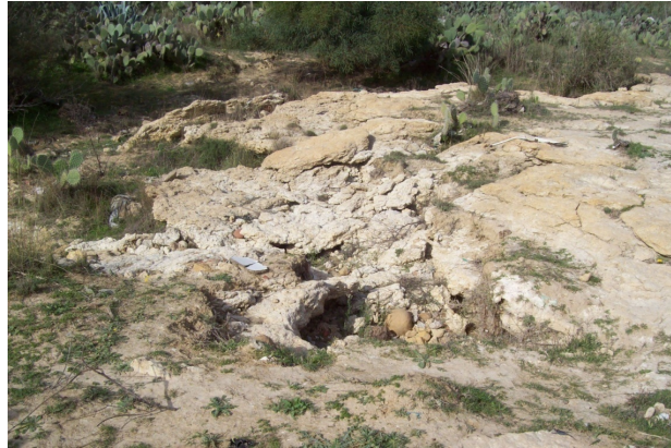
Photo 3. Fracturing and collapse of limestone crusts.
