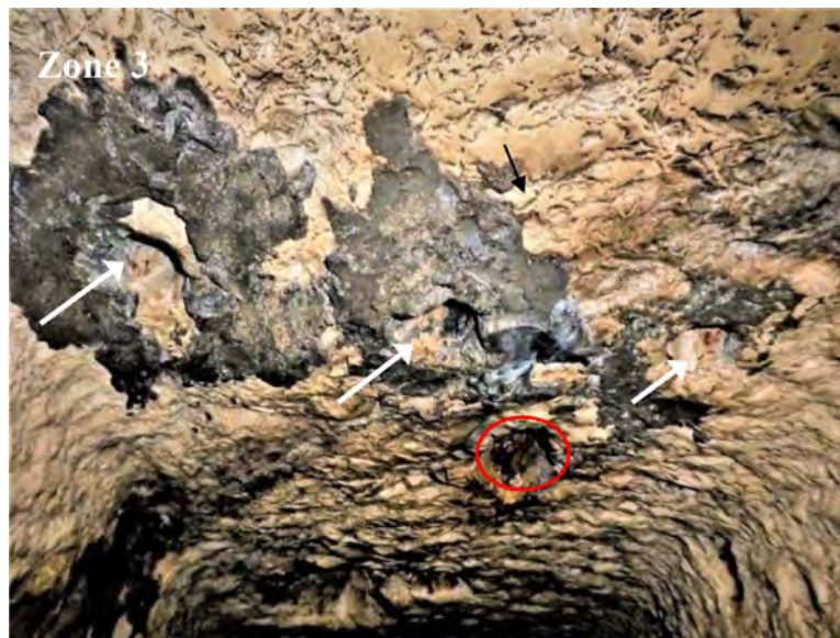
Figure 16. Tunnel ceiling, alteration Zone 3. Three hand-carved depressions (arrows) roughly encircled with a layer of black pozzolanic mortar. Another depression with a rust interior is present beneath (encircled red). (see Table 2 , Table 3 , Analyses for Zone 3).
