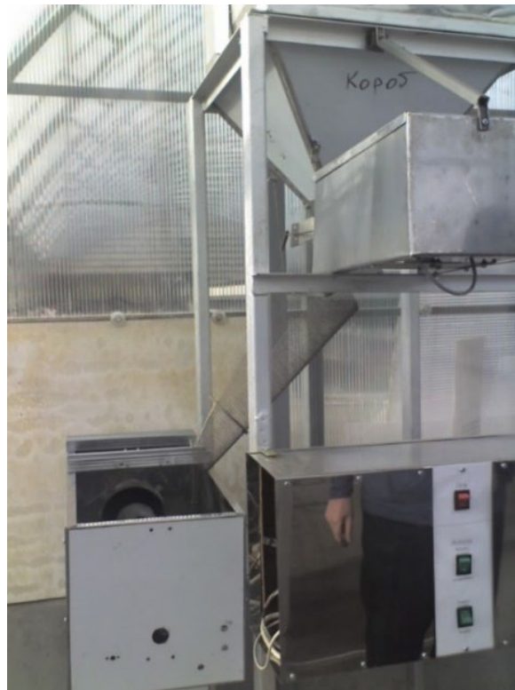
Figure 1. External view of a pellet burner unit with pellet bunker and control unit in an operating heat supply system.
