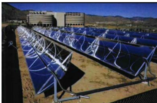
Figure 2. Solar parabolic trough power generation station was built in California desert, USA 图 2. 美国加州荒漠上建成的槽式太阳能热发电站
