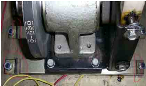
Figure 2a.The disintegration discovers to prop up steel plate to split 图 2a. 解体检查发现支撑钢板断裂
